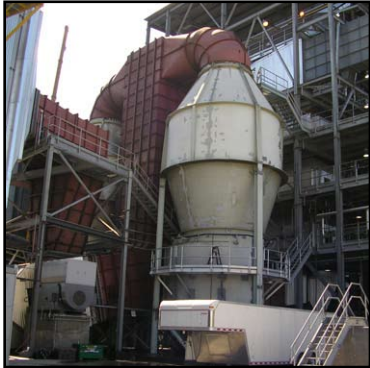
One of two scrubbers to be rescued with Belzona
