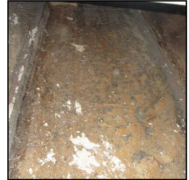
Belzona® 1391 eleven months later. Discoloration is caused by elevated temperatures but coating is 100% intact and fouling was totally eliminated
