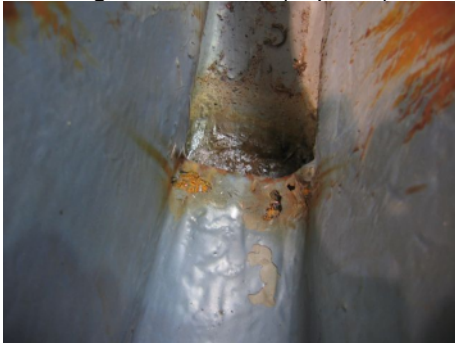
Fig 4 – Cavitation to pump cutwater
