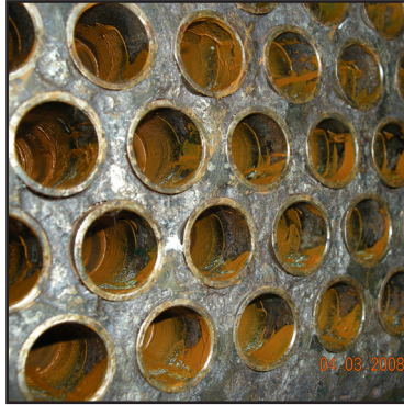
Close up of erosion on tubesheet
