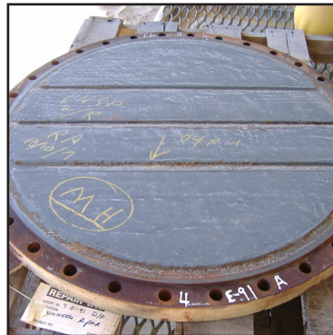
Heat exchanger after five years in service
