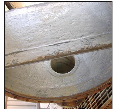
Heat exchanger channel head after five years in service
