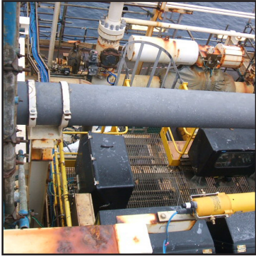
Manifold showing weathering of paintwork
