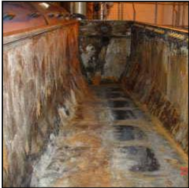
Original corroded condition
