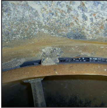
View of the gap between the tubular screw conveyor and the housing
