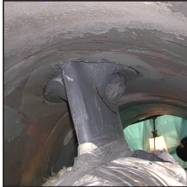
Extensive damage to Glass Flake lining (Starboard)
