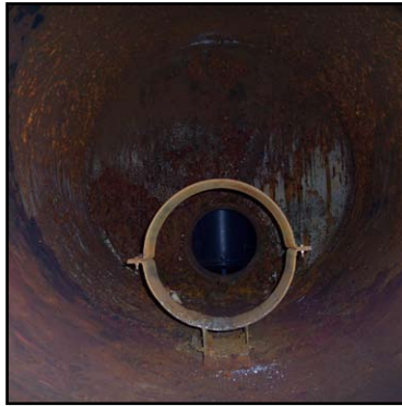
View of the internal corrosion
