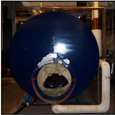
The tank inside the Powerhouse
