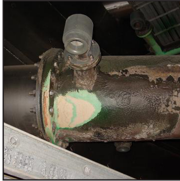
Severely damaged FRP pipe caused by lime slurry
