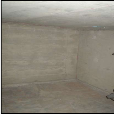
Bare unprotected mixing tank
