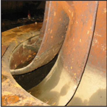
Damaged and worn runner
