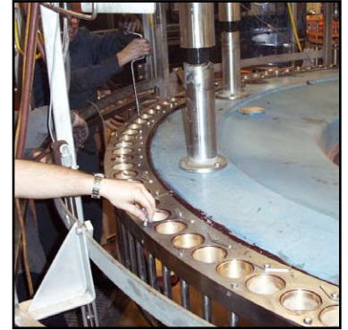
Stainless steel plates seated in Belzona for full support and corrosion protection
