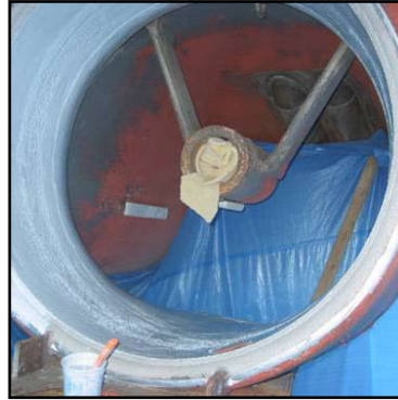
Application of first coat of Belzona® 1341 with additional coat to fill voids.
