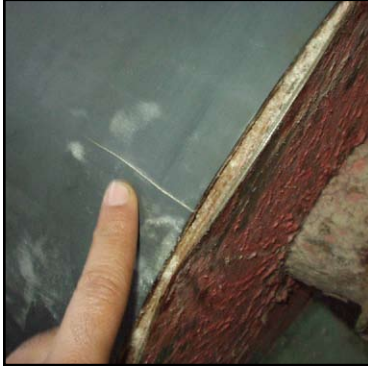
The crack in the rubber cover
