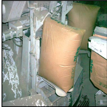
Cement packing machine.
