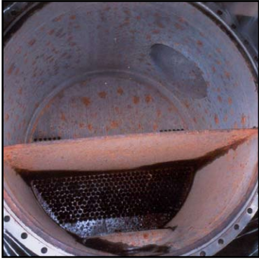
The corroded water box.
