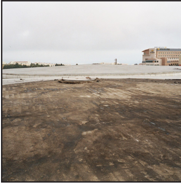
Damaged tank roof
