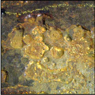
Extent of the corrosion due to the effects of the microbiological attack.
