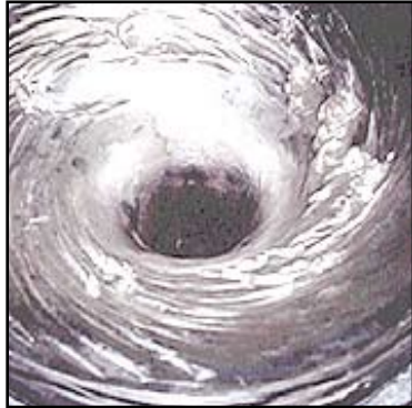
Damaged steel end plate
