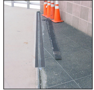
Finished joint with Belzona® 2221 and Belzona® 4411 (Note: old steel covers and tape)
