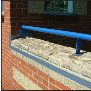
Close up of typical damaged block
