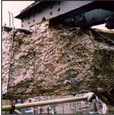
Close up of the badly spalled concrete
