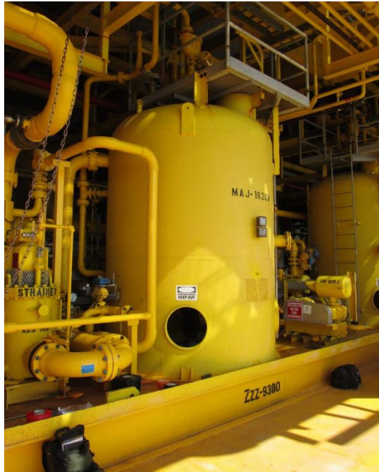
Caption: Leaking seawater filter vessel
