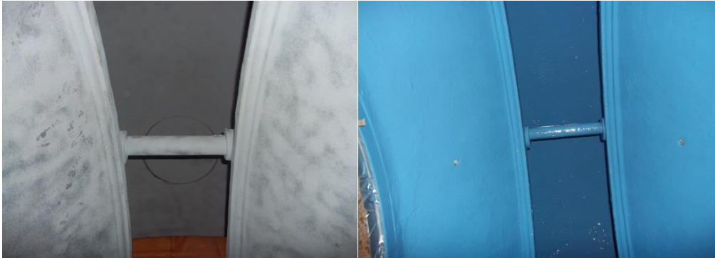
Image 11- Pump casing after Sponge Blast
