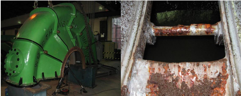
Image -2 Pump casing mounted on blocks
