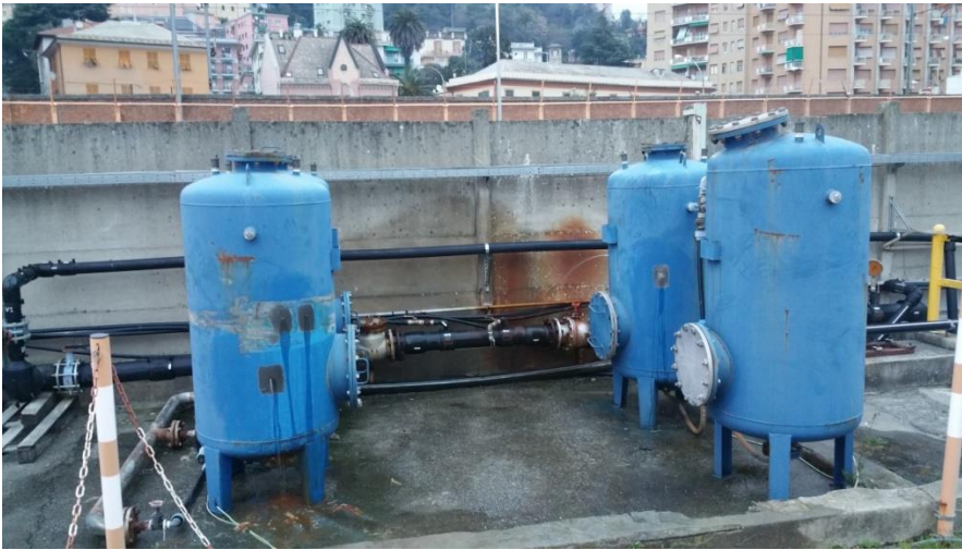
Image 1: Leaking seawater tanks at hydrocarbon storage tank farm
