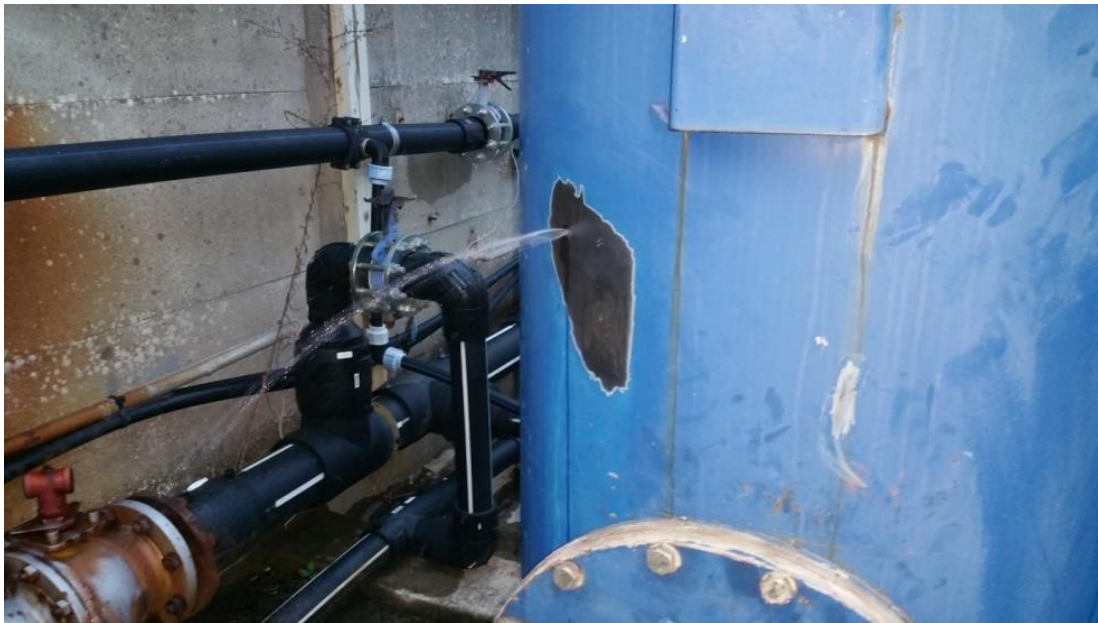
Image 2: Live seawater leak
