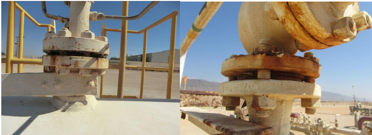
Flanges damaged by corrosion
