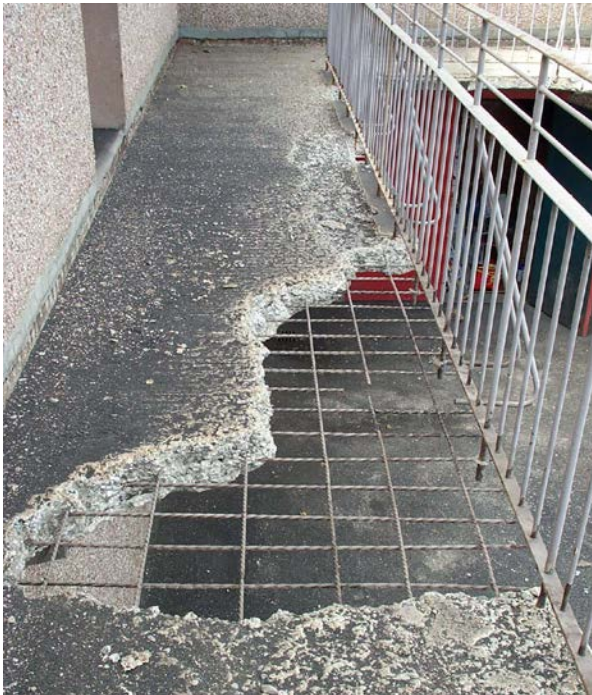
Damaged Concrete Walk Way 2002
