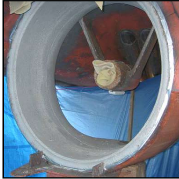
View of one of the blasted nozzles.
