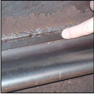
Leaking Expansion Joint
