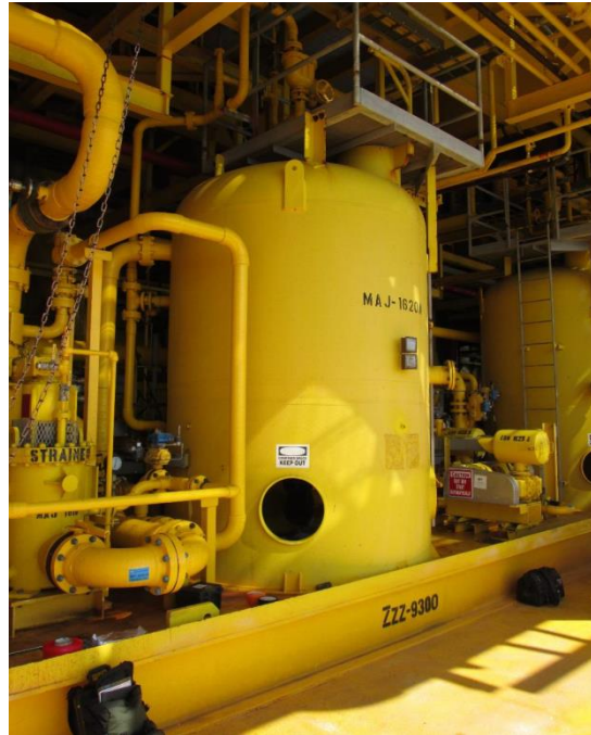
Caption: Leaking seawater filter vessel
